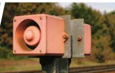
Example of a TOWS warning siren
