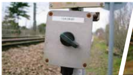
Example of a TOWS switch
